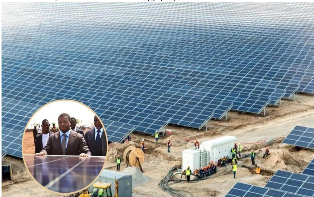
Figure 5: Togo's 50MW Solar PV Plant [23].
